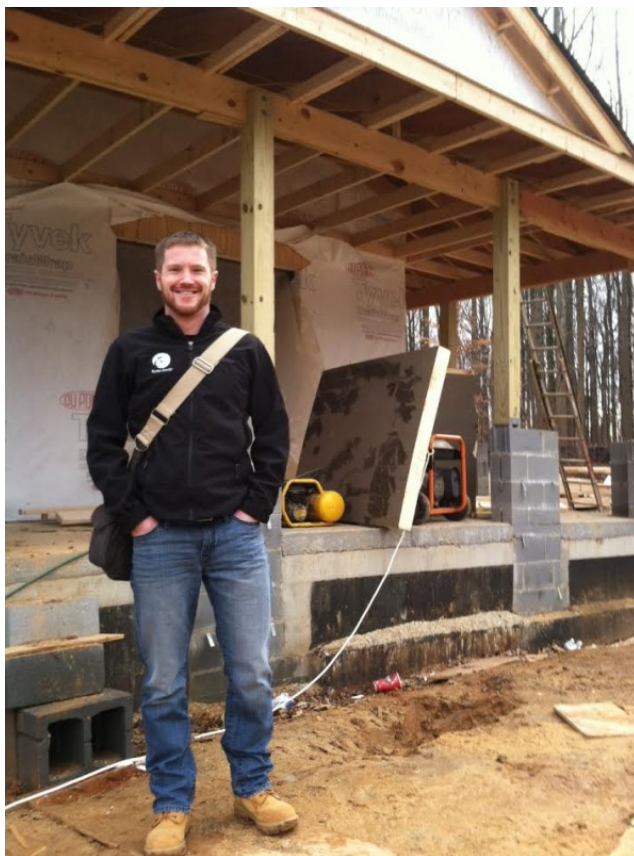
Andy Corral of Elysian Energy, getting acquainted with the project. Andy will be certifying that the work complies with Passive House requirements
