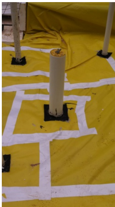
Drain, waste, and vent pipes are sealed to the 15 mil vapor and air barrier with rubber gaskets.
